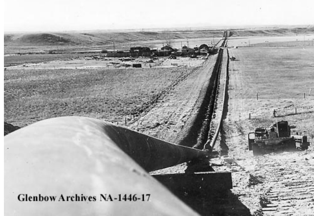
Top: Joining sections of pipeline between Turner Valley and Calgary (1920-29) Bottom: Laying gas pipeline between Carbon and Calgary 1958. Images courtesy of the Glenbow Archives.
